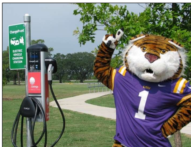
Charger installed on the Louisiana State University campus. Photo from Louisiana State University
